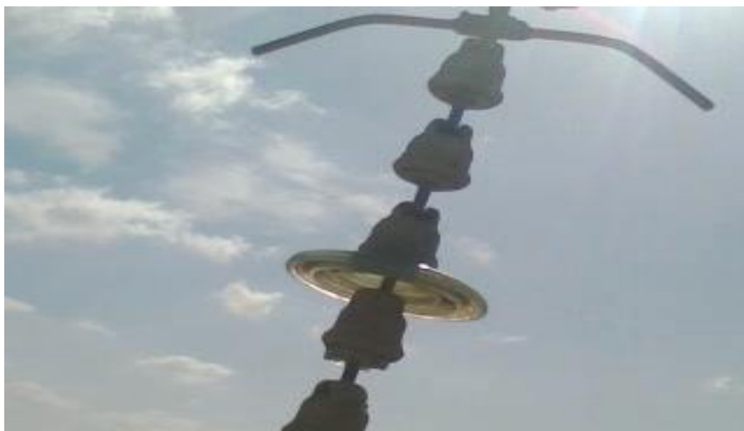
Broken glass insulator
