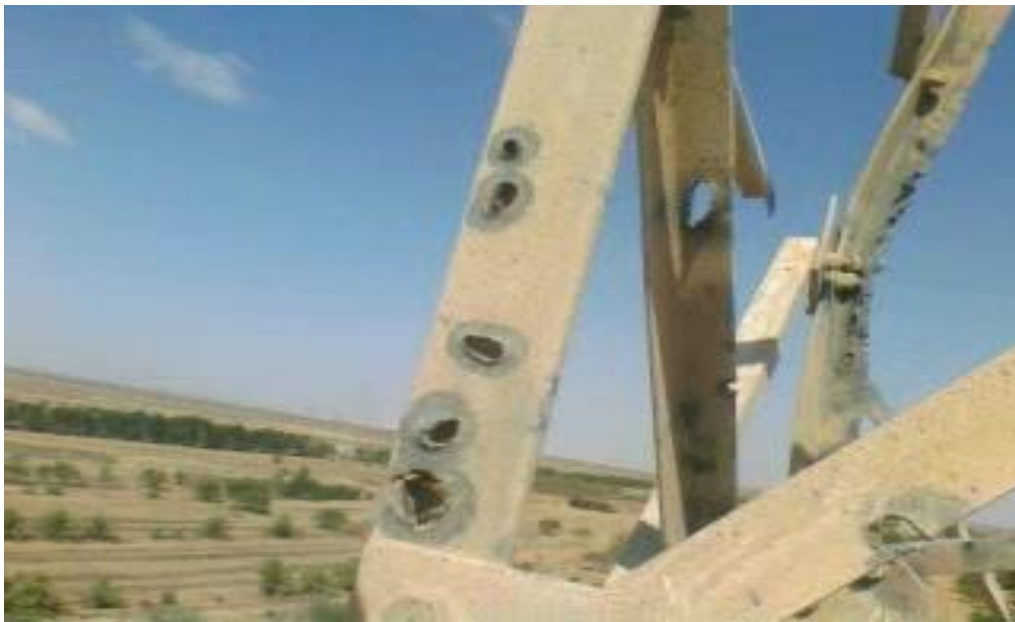
Defected steel members
