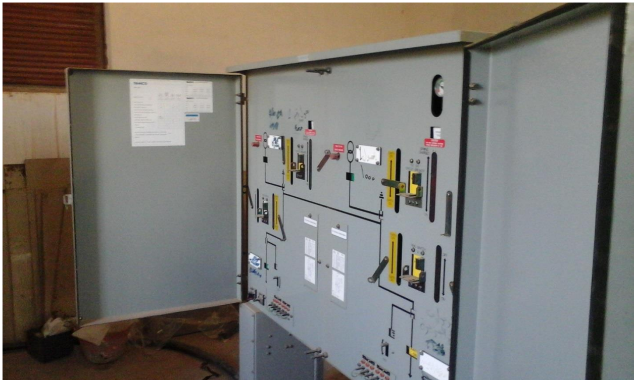
Meduim voltage GIS ring main unit
