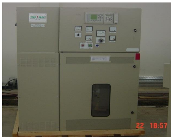
Medium voltage panel
