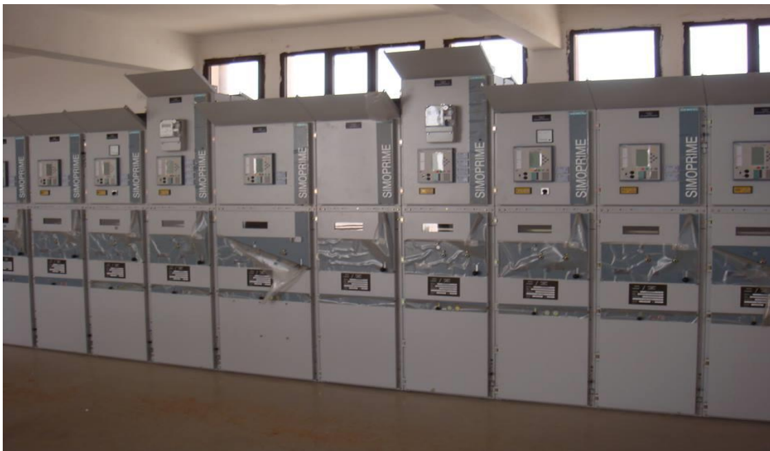
Medium voltage distribution panels (Siemens)
