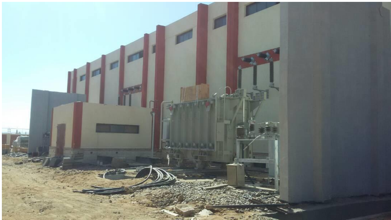
Gehena 66\11 kv substation (Sohag-Egypt)
