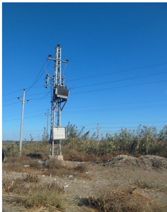
Pole mounted transformer
