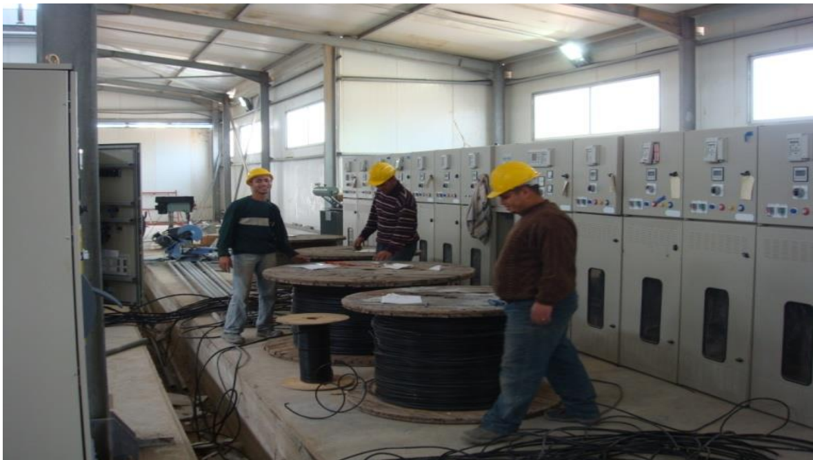
66/11 kv AIS indor substation (Elnoor ,albidaa, libiya)
