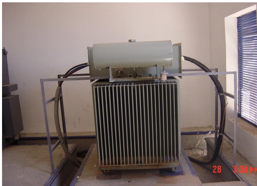
Meduim voltage transformer
