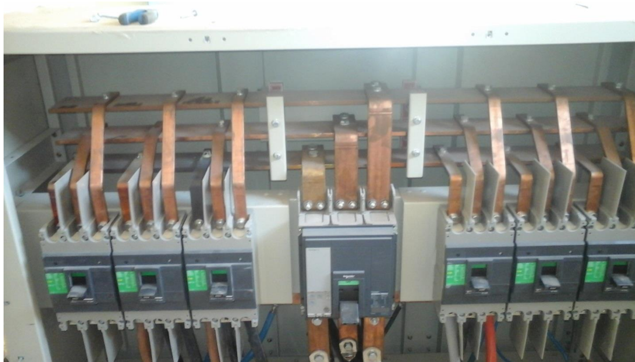
Meduim voltage distriution panel
