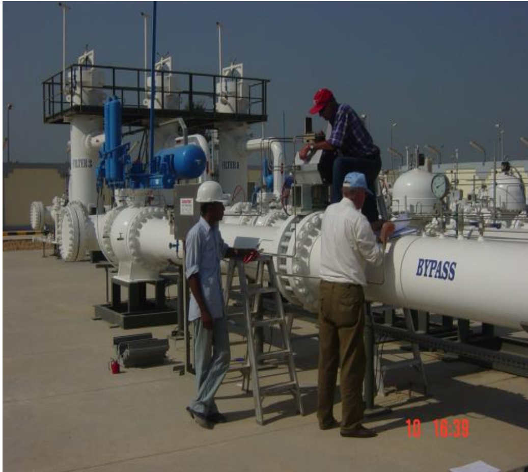
Nobaria Power Plant Gas Station
