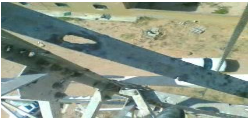
Defected steel members
