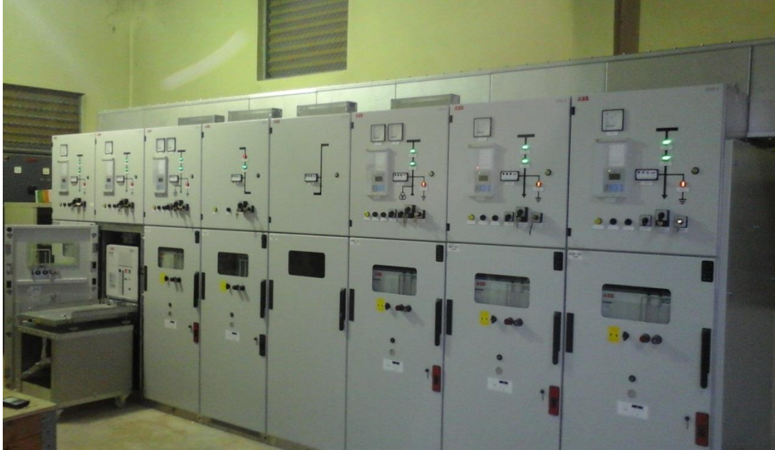
Medium voltage distribution panel (schneider)
