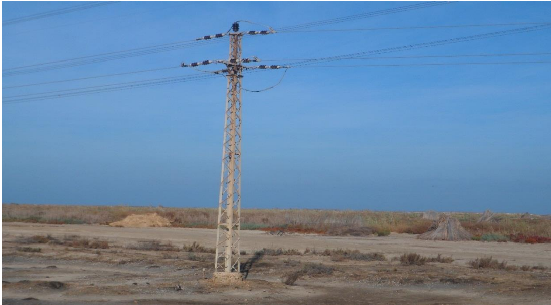
11 kv tension poles
