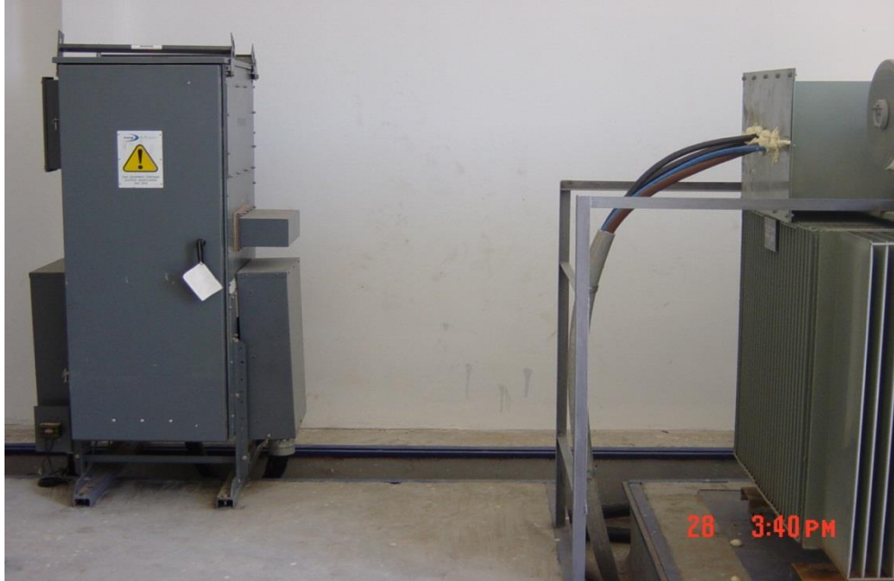
Meduim voltage distriution sustation
